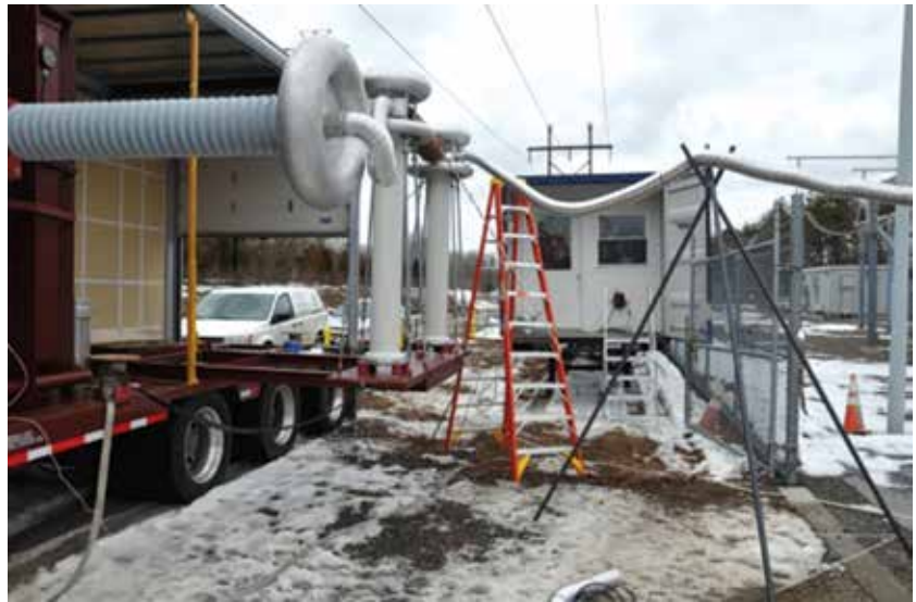
Phenix's mobile 16 MVA system setup to test 138 KV superconductor transmission cable with optional partial discharge measurement.
