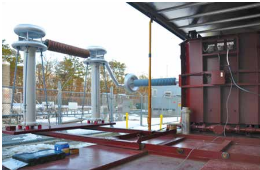
Phenix's mobile 16 MVA system testing 138 KV superconductor transmission cable.
